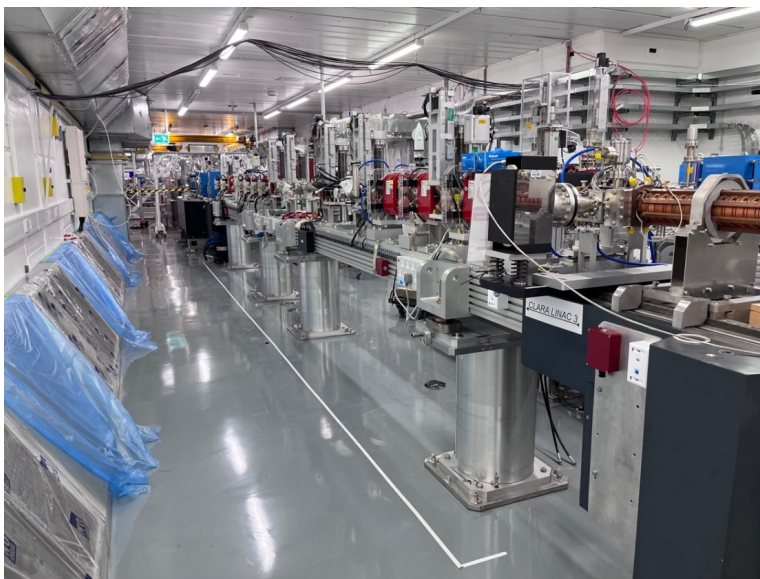
CLARA upgrade installation showing part of linac and beamline including variable bunch compressor dipoles (in blue) at the far end.
